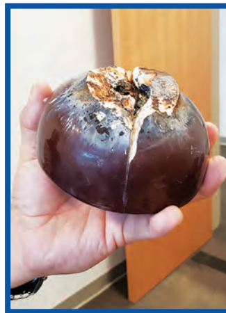
Broken insulator likely damaged by a lightning strike.
