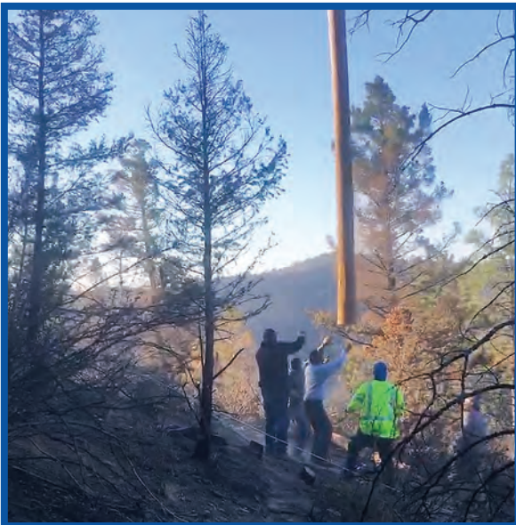
Crews reach up to steady a pole lowered by helicopter and place it in a hole prepared for its setting - one of 26 poles replaced as a result of the Rio en Medio fire which started several miles away from JMEC lines.
