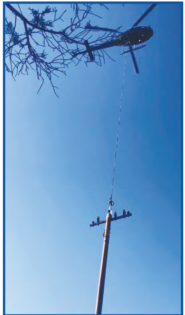
Some areas in JMEC service territory are so remote pole replacements have to be helicoptered in.
