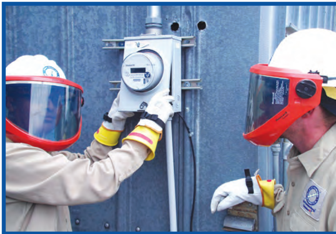
Meter readers Jesus Guzman, (left) and Josh Bakken install one of the more than 30,000 new meters going in throughout JMEC's system in the coming years. The new meters provide more and immediate information about quality of voltage and outages.
