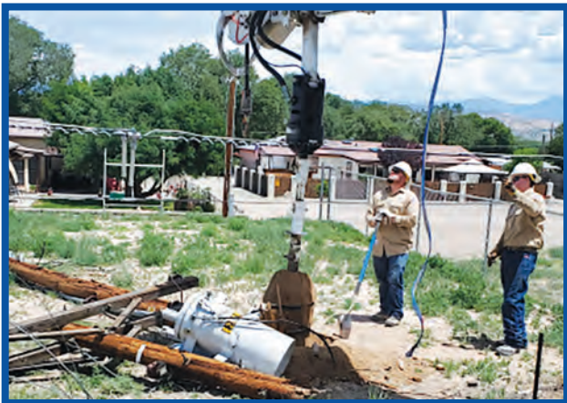
JMEC crew members Pat Archuleta, left, and Walter Bustos work on replacing a pole that was broken after a lower hanging wire was caught by a vehicle.
