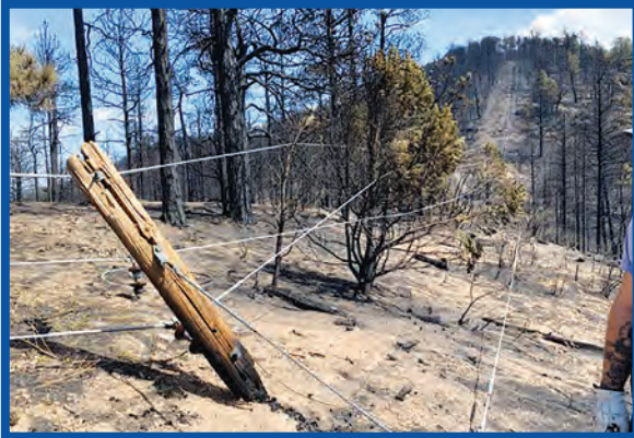
The Rio en Medio fire, started some miles from JMEC lines, burned poles from the bottom up so, all that is left holding it together are the lines.
