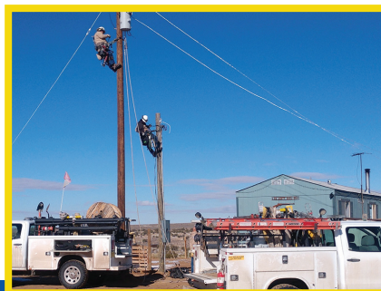
Tall pole, Darren, JMEC journeyman lineman; shorter pole, Jacob, JMEC journeyman apprentice; bring power to this Navajo Nation home.
